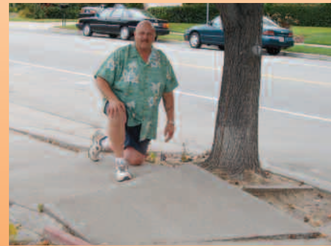
Dion is seriously concerned about the deteriorating condition of Gilroy's sidewalks and determined to see that something is done about it.
